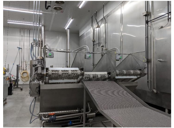
Conveyor off of three lane chiller
